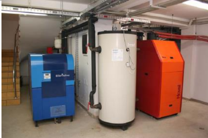
Picture 1 Adsorption chiller and pellets boiler
